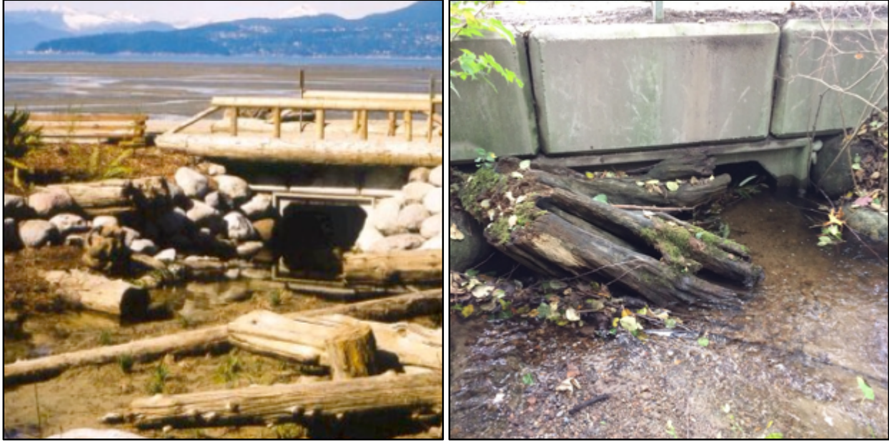
Figure 18: The lower reaches of Spanish Bank Creek have been filled with sediment. Installed in 2000, the concrete box culvert pictured above is 6 m long, 1.2 m tall, and 1.8 m wide (left; Hollick-Kenyon, 2002). After 16 years only a fraction of the culvert is passable due to build-up of sediments (right; Reynolds, 2016).
