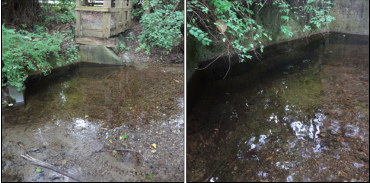
Figure 19: A pre-cast concrete headwall was installed at Spanish Bank Creek. The pre-cast concrete headwall is located at the north end of the wood stave culvert that spans under NW Marine Drive (left). Accretion of sediment has filled in the lower reaches of Spanish Bank Creek, thereby impeding flow through the wood stave culvert (right; Reynolds, 2016).
